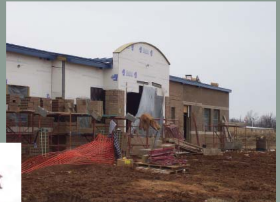
Pictured above is the front of Clever High School while under construction. At left is the completed facade of the new Clever High School, dedicated in August 2008.
